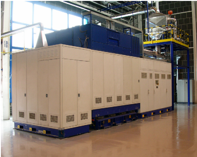
Fig. 1. Picture of the SOFC CHP test site in GTT (Torino, Italy).
